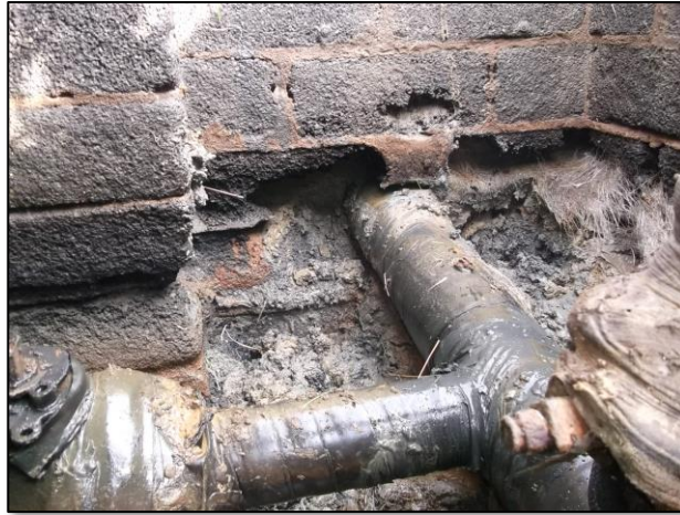
Figure 10 - Evidence of valve chamber degradation, replacement and valve/pipework refurbishment
