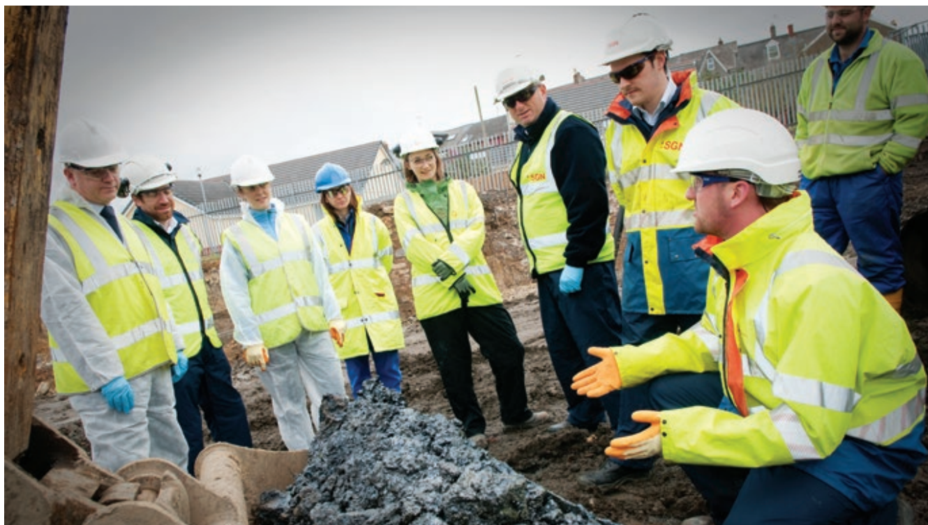
Representatives from other UK gas distribution companies visited our land remediation project at Pembroke Dock
